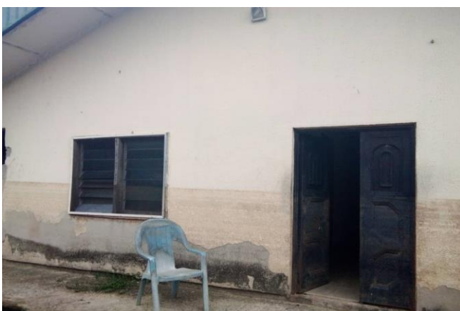
Figure 17.0: Flood mark on Residential Building in 2018 flood level mark in Otiokpoti, Ogbia Local Government Area.
