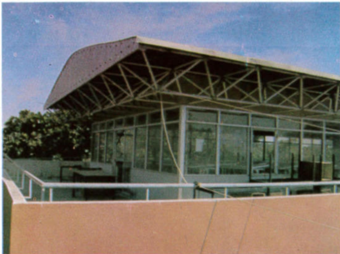
Plate 14. Roof-top Studio, Department of Architecture, Ahmadu Bello University, Zaria. The pitched roof was constructed on top of the space truss originally covered by plywood boards. Source: Photograph by the authors (November 2005).
